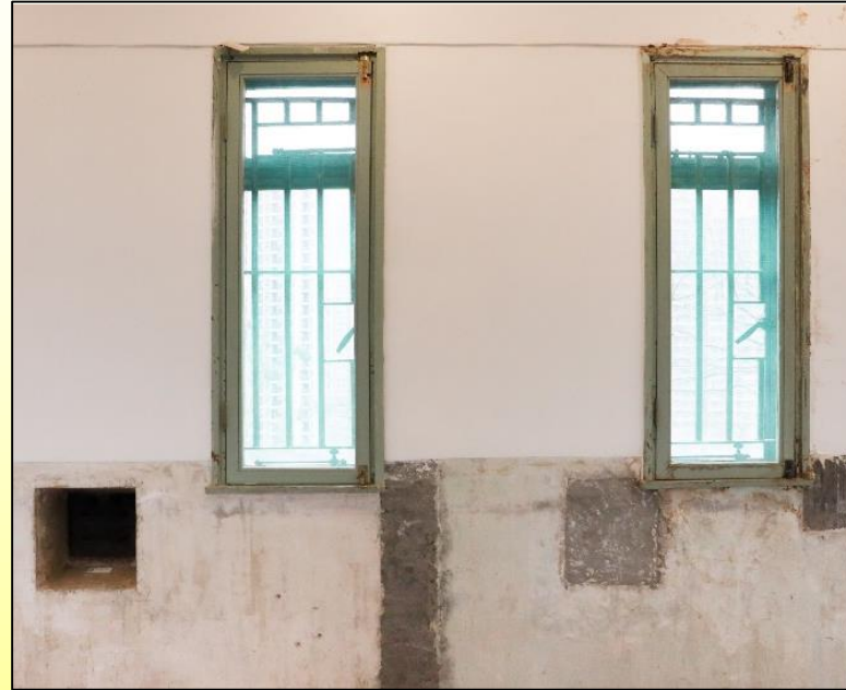
裝有木框和金屬窗花的舊窗被保留 Old windows, fitted with wooden frames and metal grilles preserved 2026 (Source: AMO)
